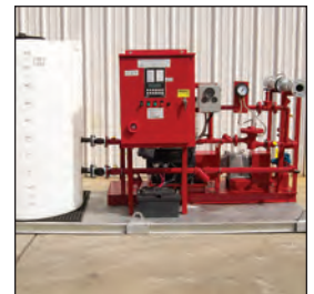
Diesel Pump Skids
