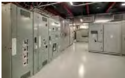
ELECTRONIC CONTROL EQUIPMENT
